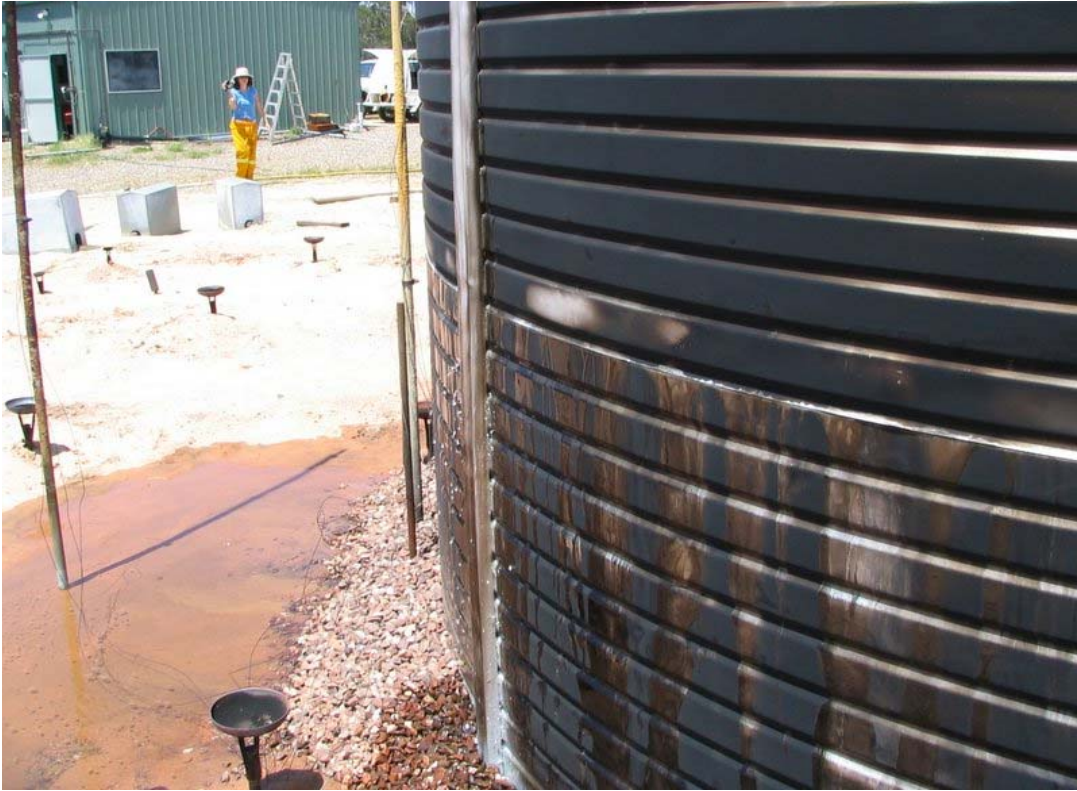
Figure C66 Bladder tank leaking and join damage as a result of structural exposure.
