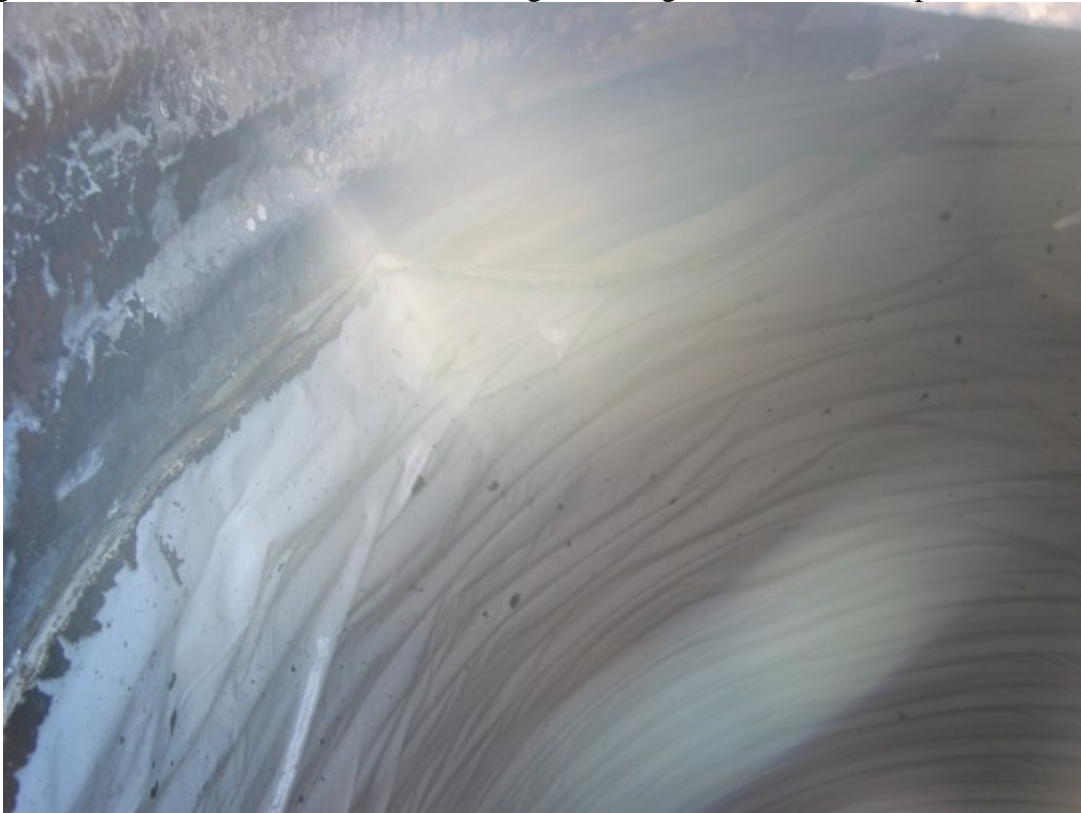
Figure C39 Tank 7 severe internal damage resulting from structural exposure.
