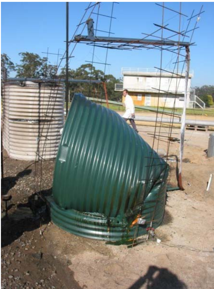
Figure 22 Experiment 14 - Structure exposure on polyethylene and metal tank
