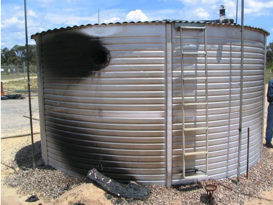
Figure C62 Damage to bladder tank overflow resulting from pre-radiation and flame exposure.
