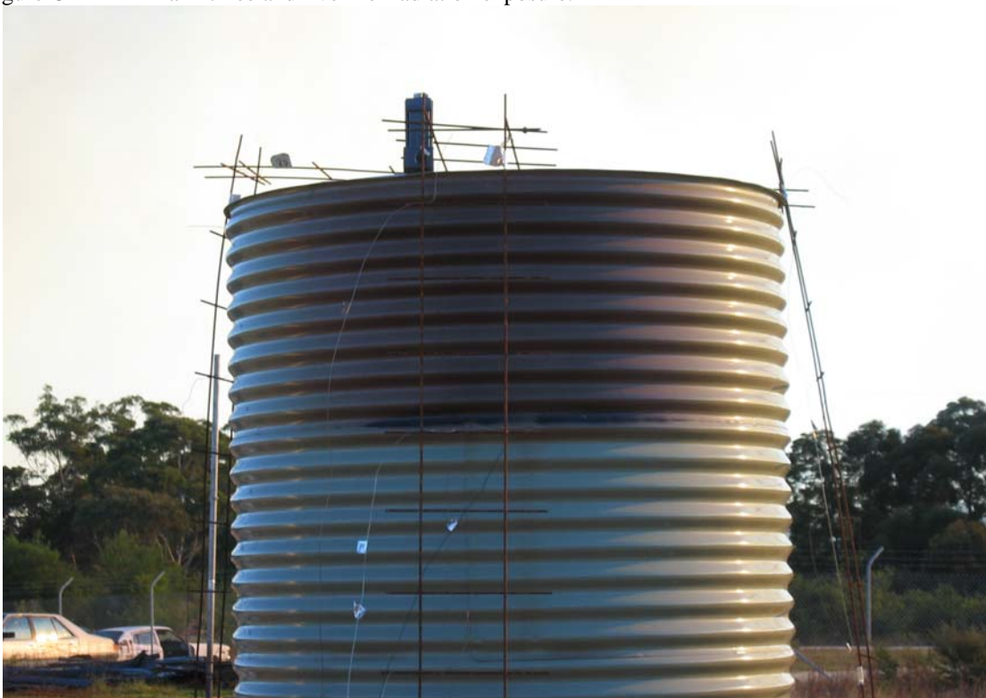
Figure C15 Tank three scorch mark above the water line.
