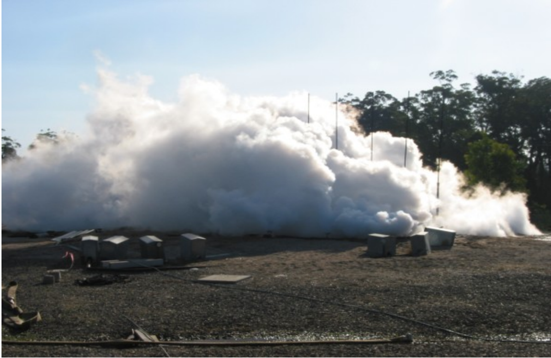
Figure C31 Tank four complete failure due to structural exposure. Escaping water extinguished gas burners.
