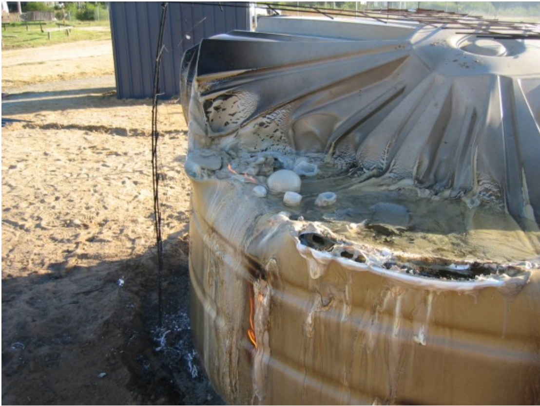
Figure C11 Tank six server structural damage down to water level as a result of per radiation exposure.
