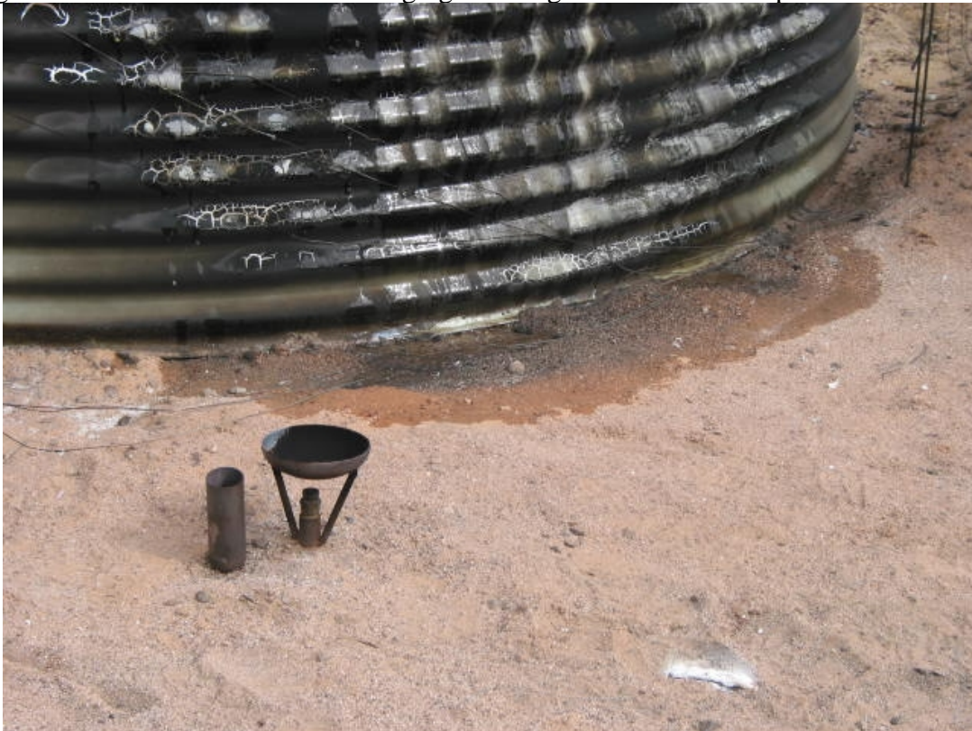
Figure C6 Tank one leaks resulting from severe damage during structural exposure.
