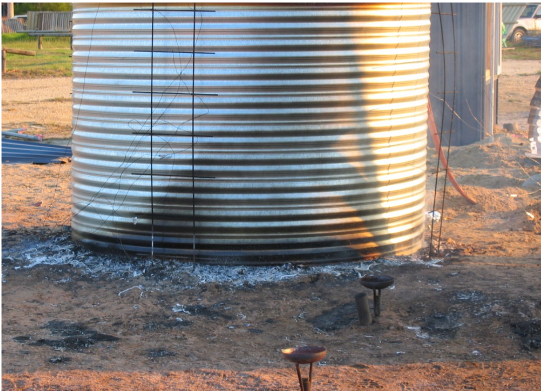
Figure C17 Tank five minor scorching from litter ignition.
