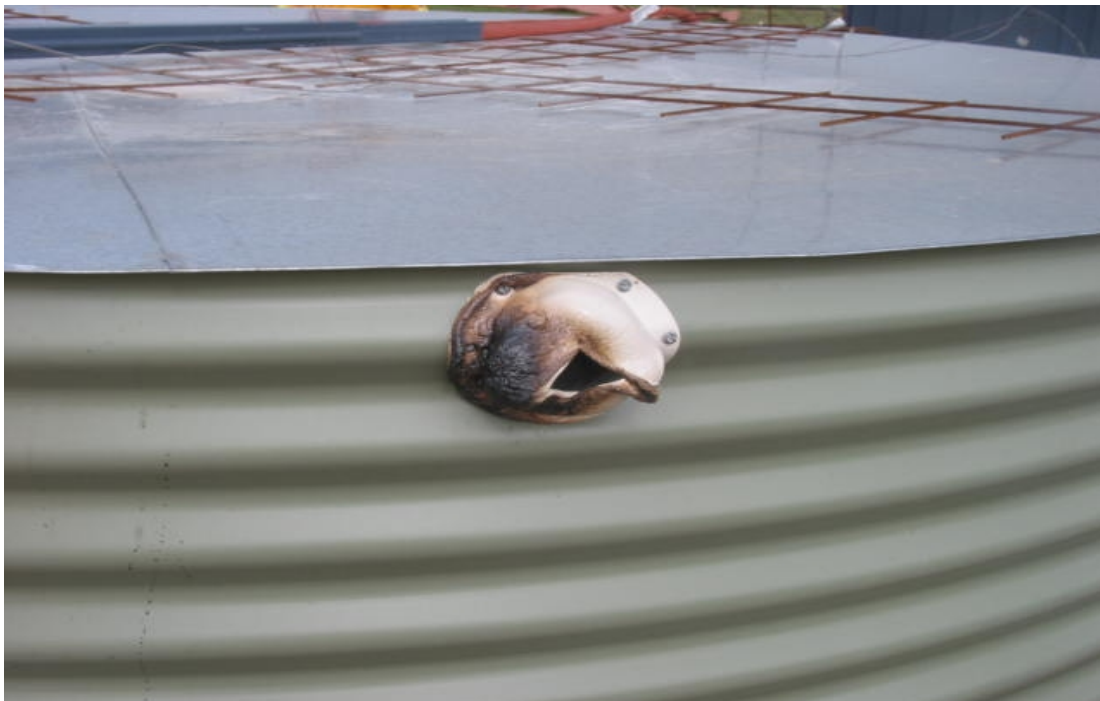
Figure C3 Tank one with damaged over flow outlet.
