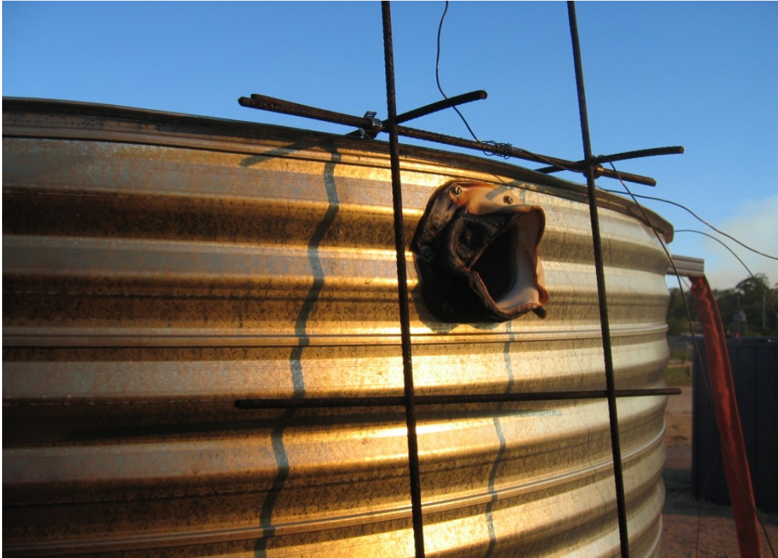
Figure C18 Tank three overflow outlet damage.
